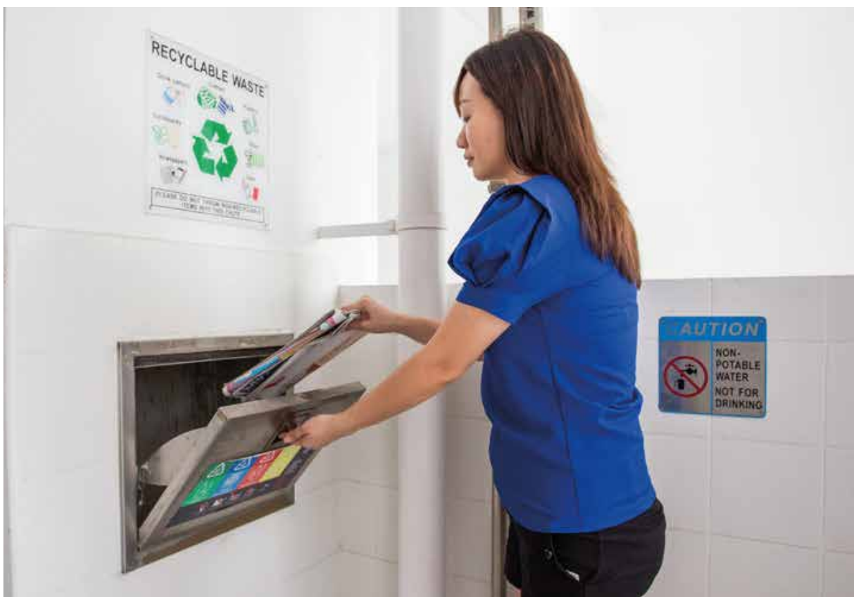
Separate chutes for recyclable waste
