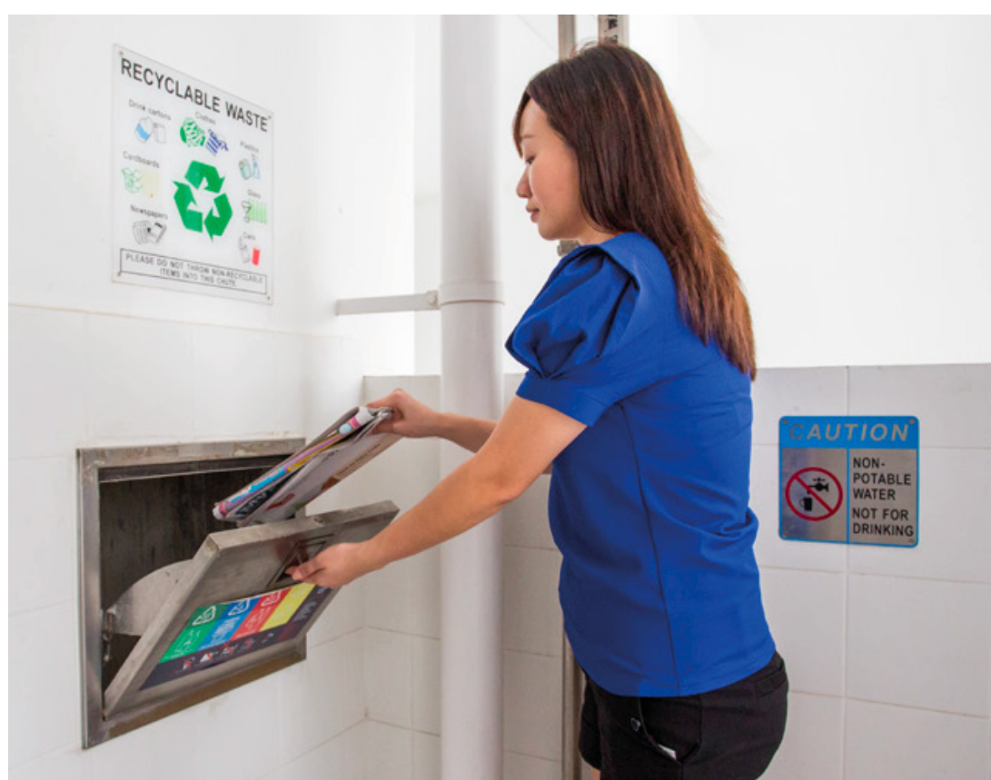
Separate chutes for recyclable waste
