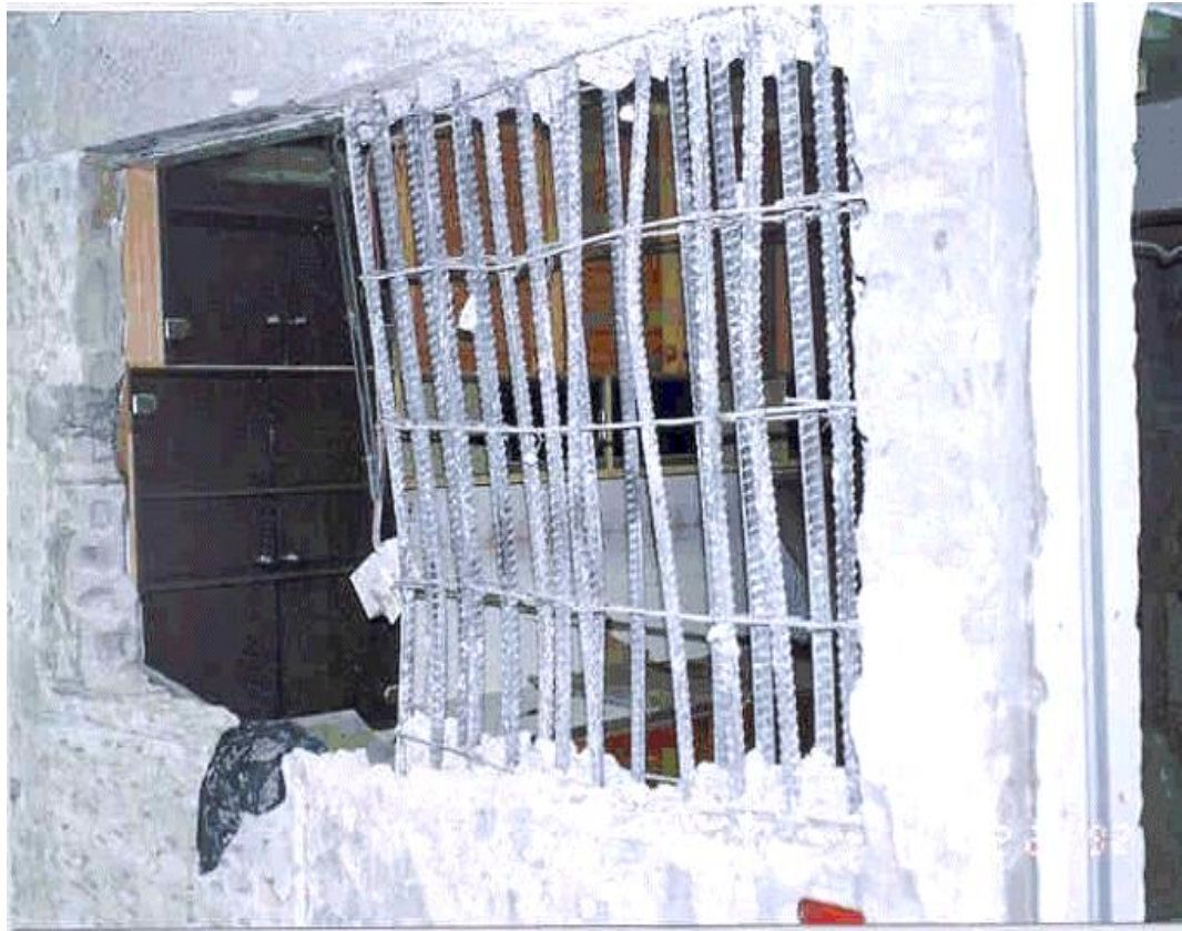
Exposed reinforcement bars
