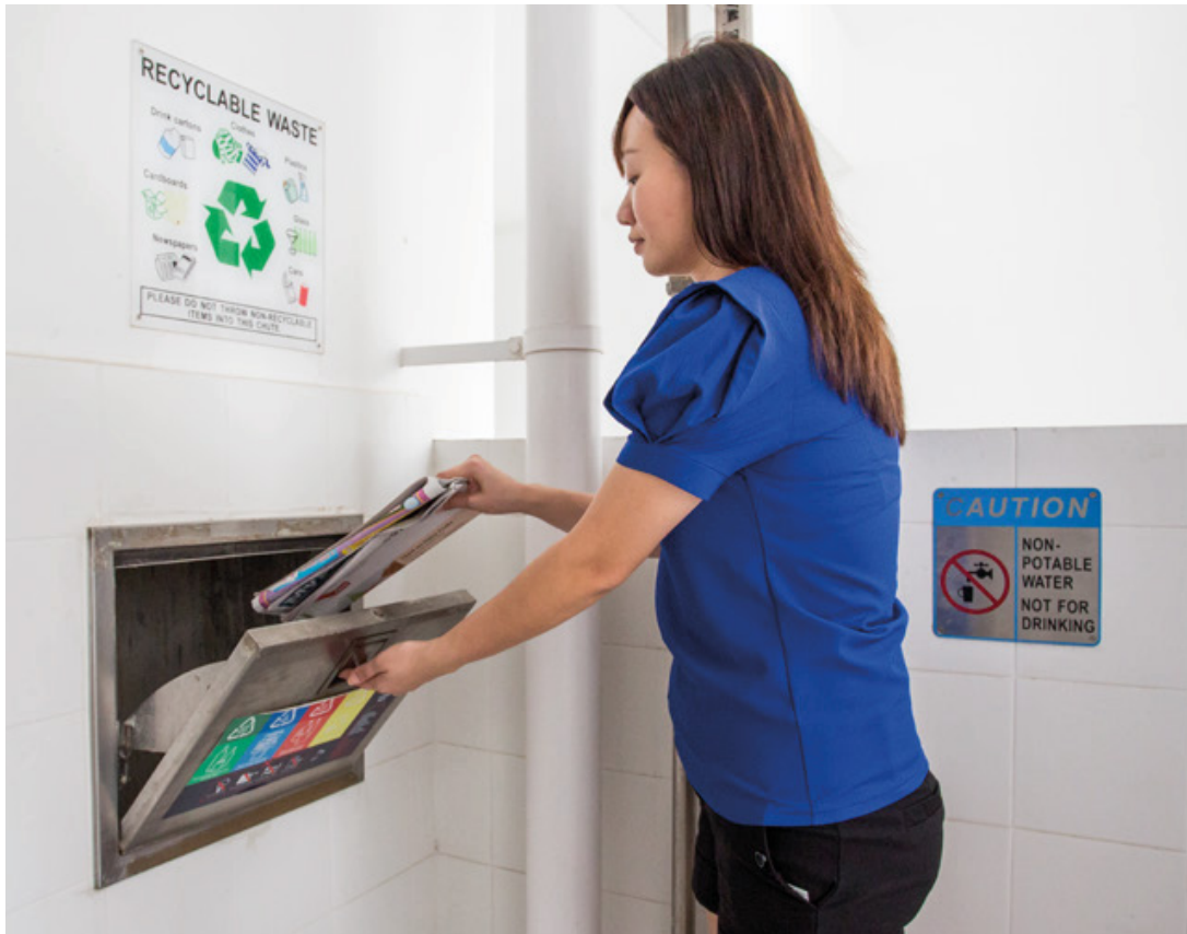
Separate chutes for recyclable waste
