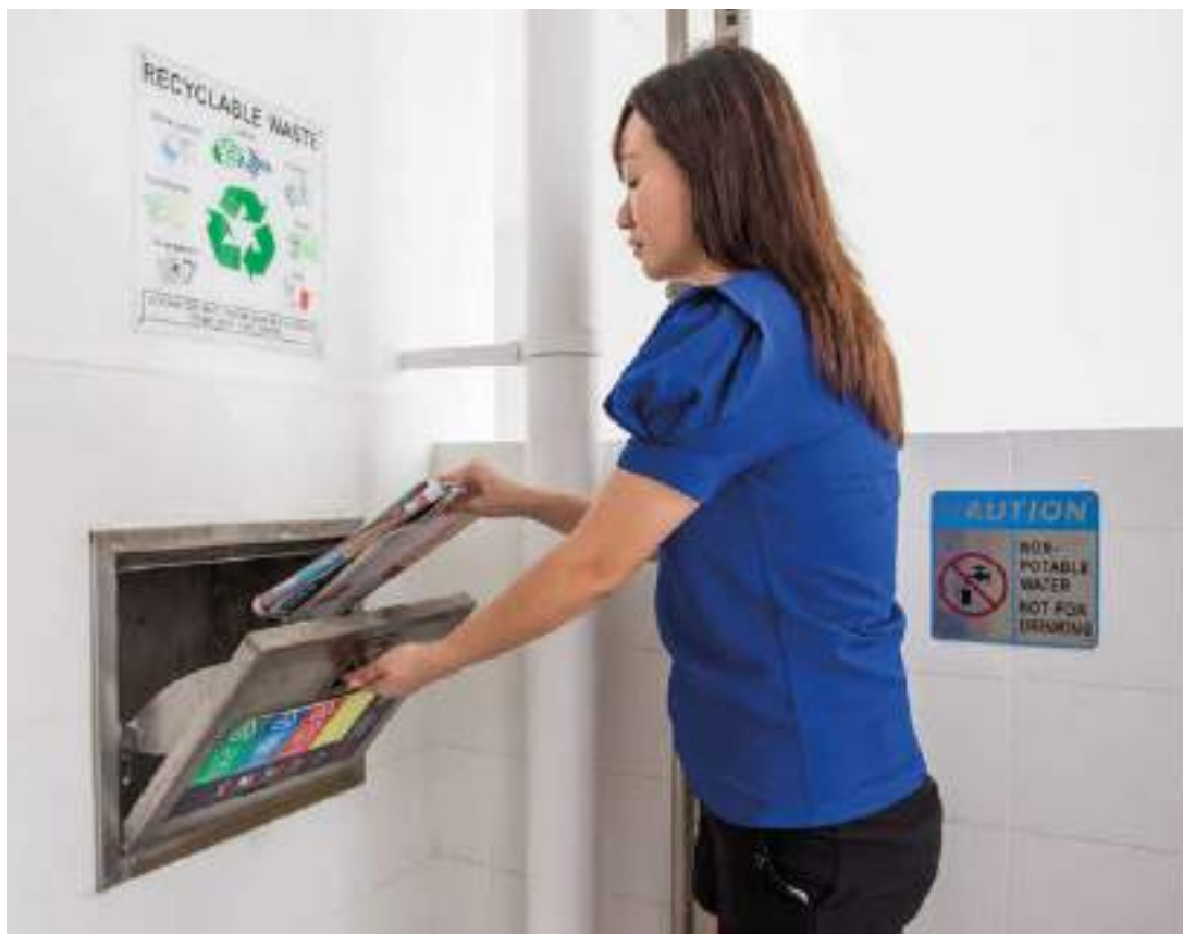
Separate chutes for recyclable waste
