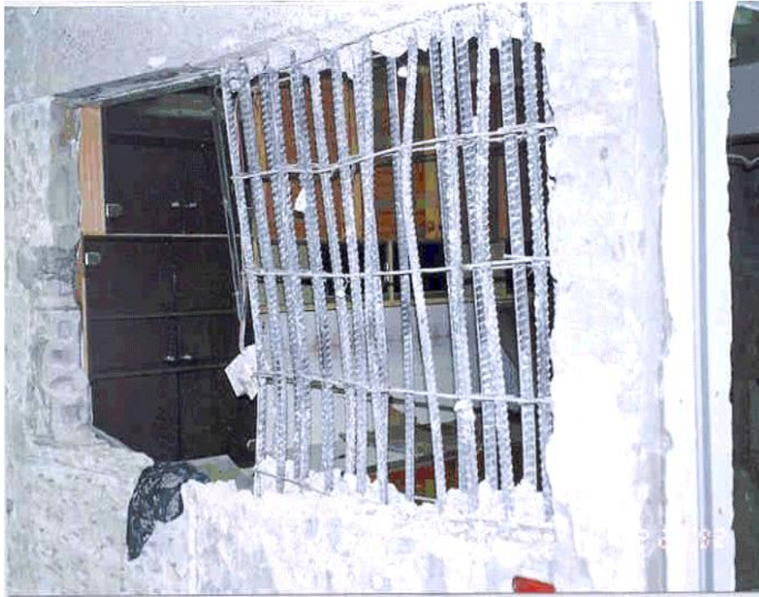
Exposed reinforcement bars
