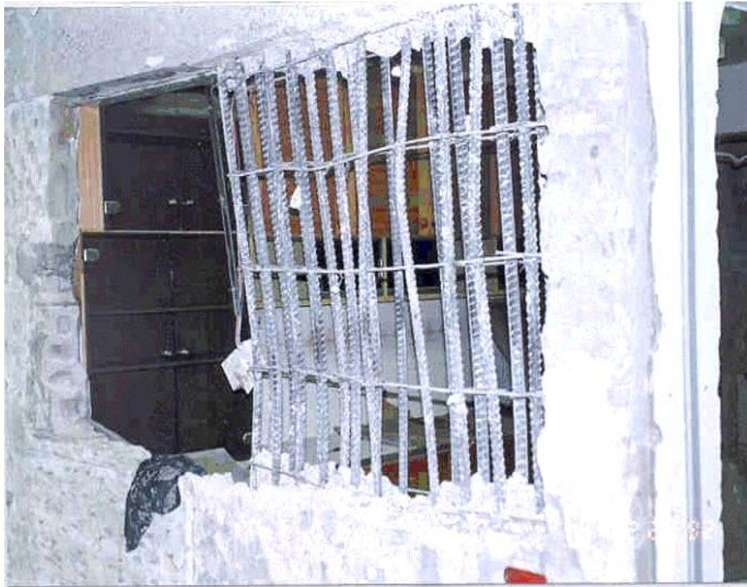
Exposed reinforcement bars
