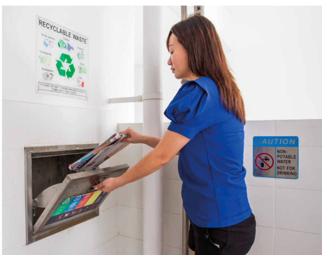
Separate chutes for recyclable waste
