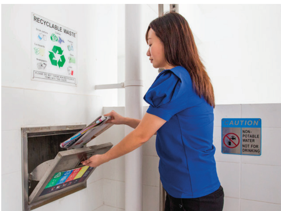
Separate chutes for recyclable waste
