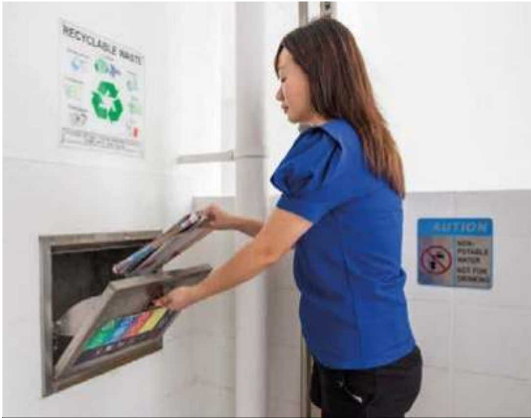
Separate chutes for recyclable waste
