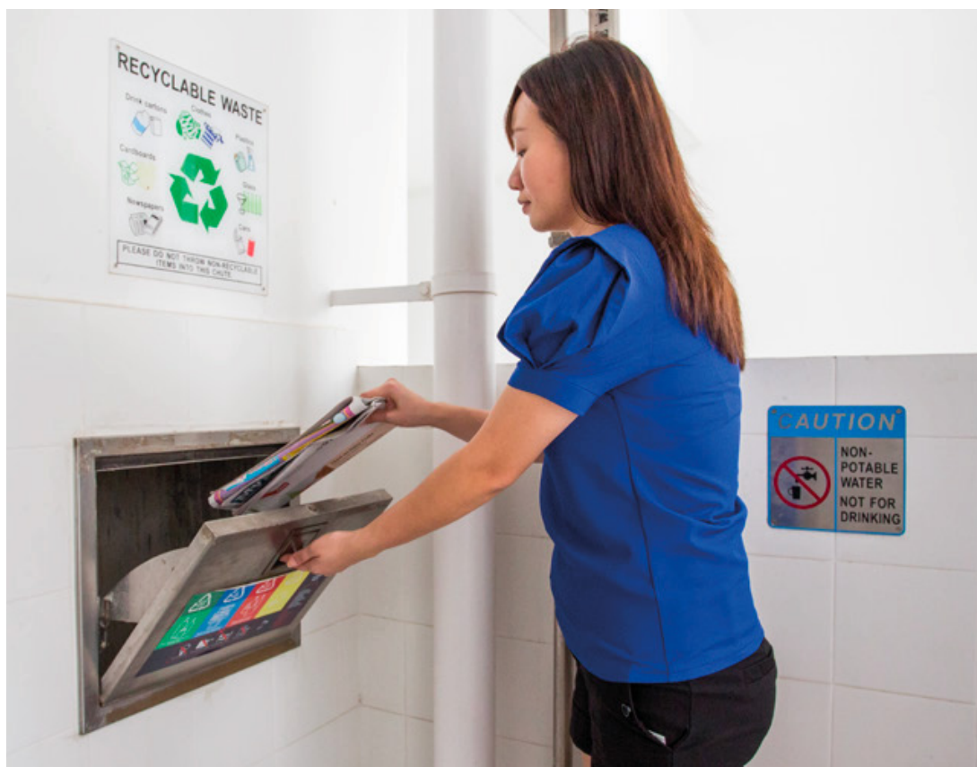
Separate chutes for recyclable waste
