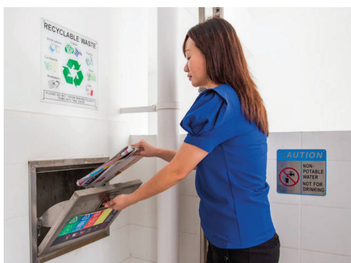
Separate chutes for recyclable waste
